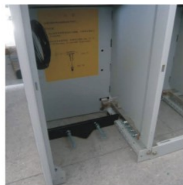
After head damper is removed
